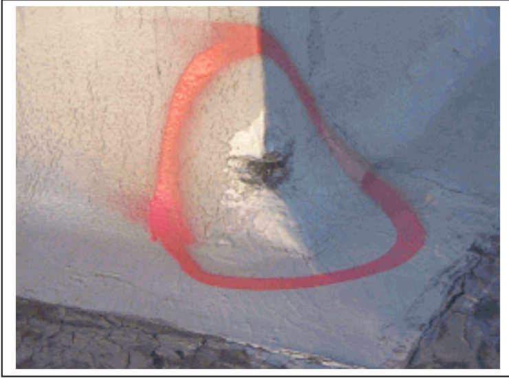
Photograph 1-Rope cut in flashing
