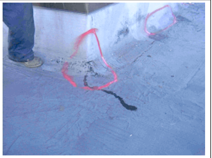
Photograph 2-Water trapped behind flashing
