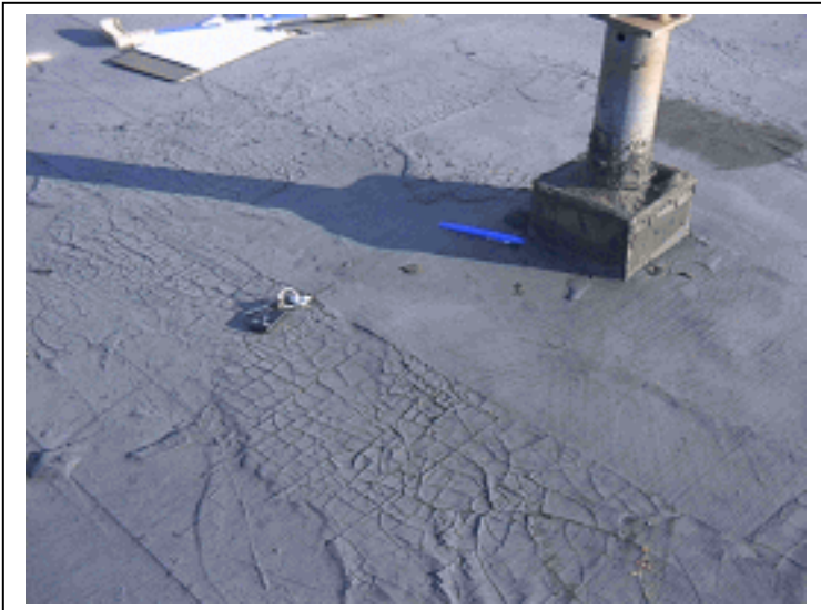
Photograph 3-Penetrations at pitch pocket stripping
